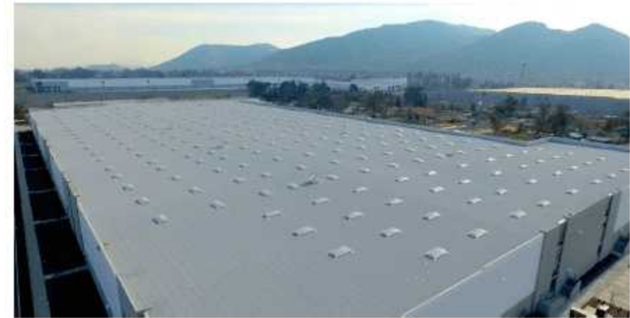
Images: Oakmont Logistics Center, Fontana, CA. 300 SKYPRO 4x8 Unit Skylights. Contractor: Mille & Severson
