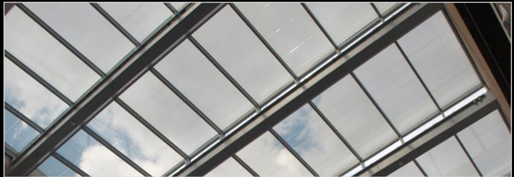
PV Skylight. 20% Semitransparent. View from the interior.
