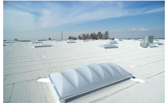
Image 3: Pictured here is a parabolic shape example. The parabolic dome is ideal for adding strength and optimizing sun light collection at all hours of the day.
