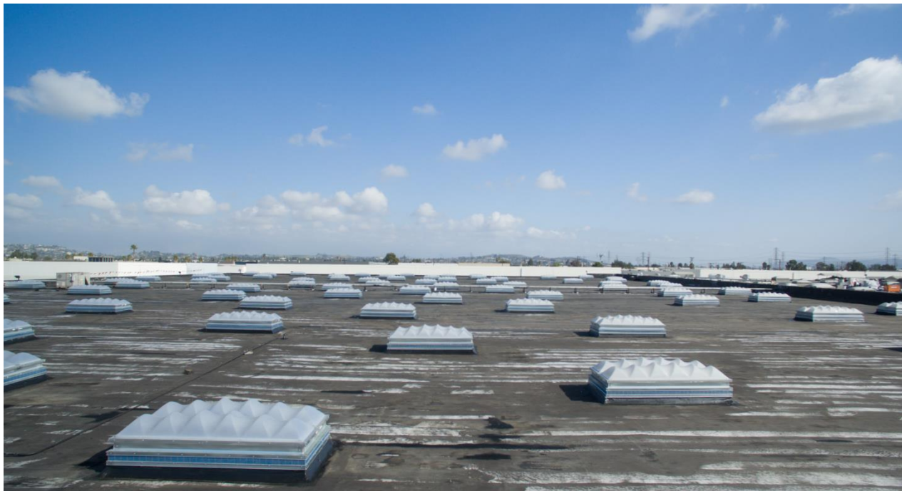
295 New UL Listed Smoke Vents by SKYCO Skylights replaced existing industrial skylights just before final elastomeric coat was applied.
